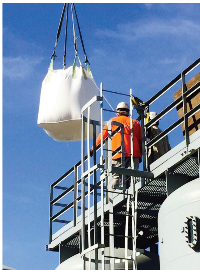
Figure 2: Workers prepare to empty a bag of IX resin atop a resin vessel at a power station.
