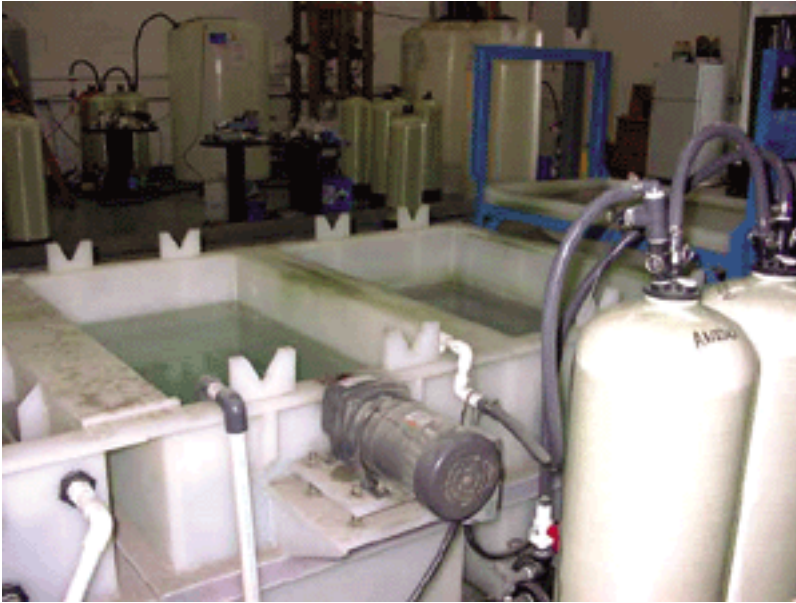
A typical dual-bed deionization system recirculating process rinse water.
