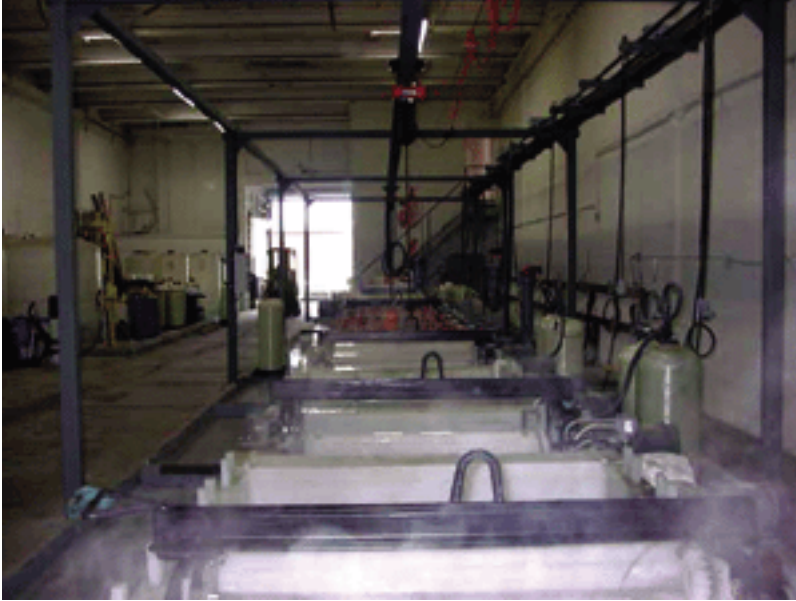
AA's system is designed for zero discharge from the plating line rinse tanks.
