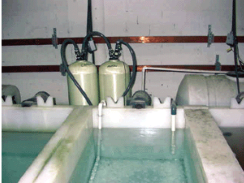
Special techniques are used at American Ammunition to minimize DI water consumption and wastewater.
